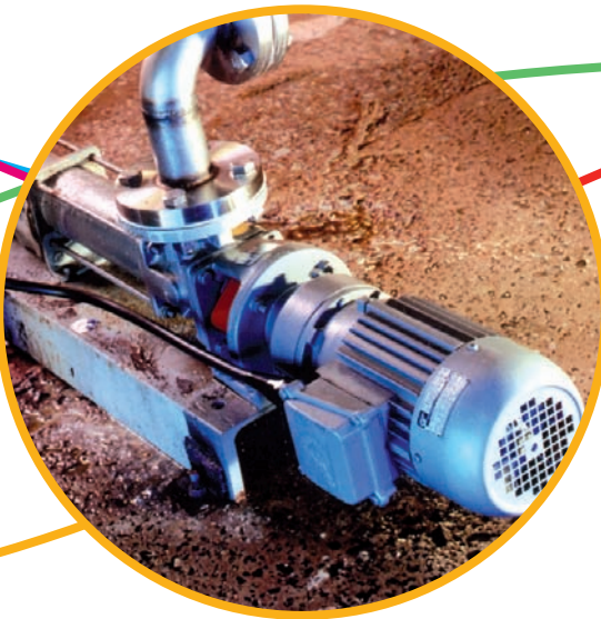
Transfer of industrial detergents
